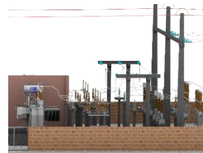
Conventional Substations Up to 550 kV
